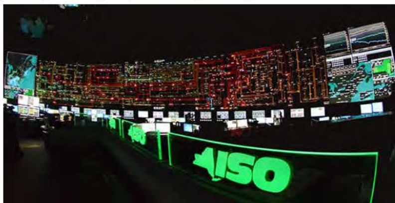
Figure 3: NYISO Control Center 8
