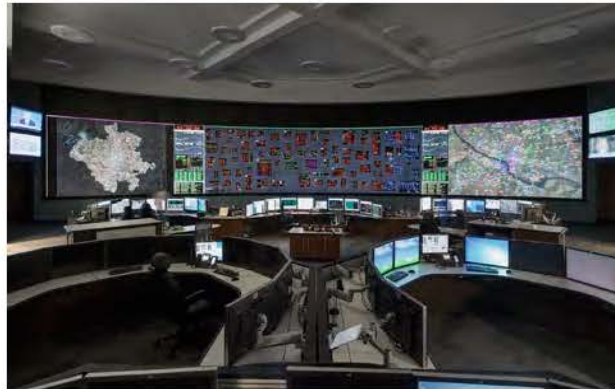
Figure 4: Austin Energy's Distribution System Control Center 9
