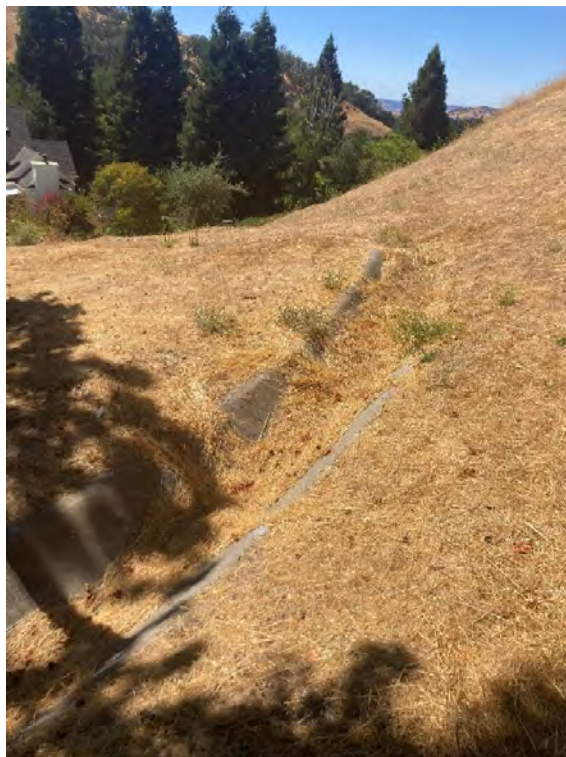
Photo 22. View of vegetative debris in v-ditch.
