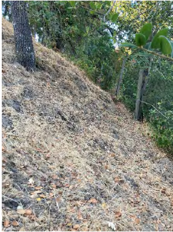
Photo 13. View of creeping soil impacting fence line.
