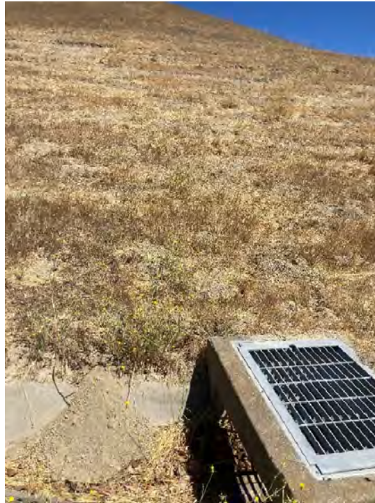
Photo 1. View of soil creep and rodent burrows on the previously graded slope above Brightwood Circle.
