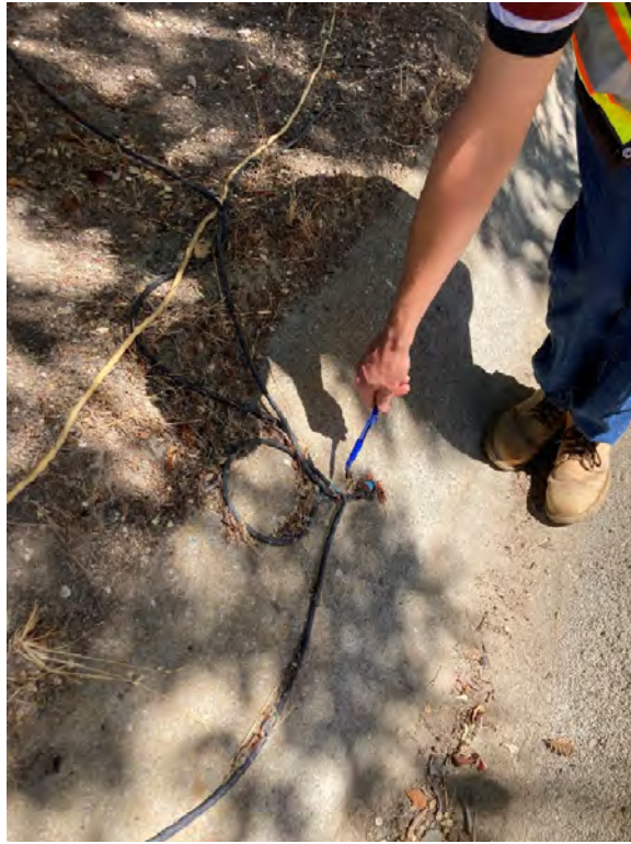
Photo 31. View of exposed wiring in v-ditch behind 102 Shadewell Drive.
