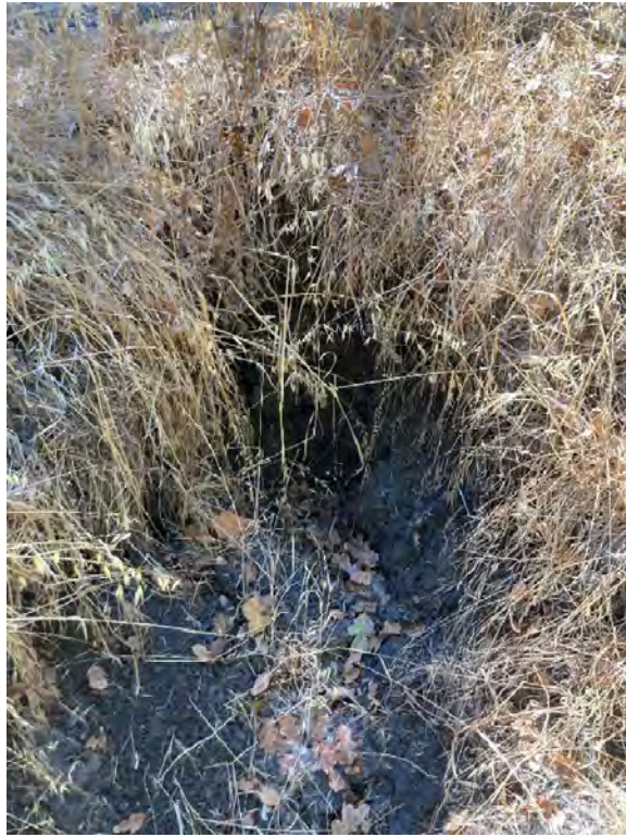
Photo 29. View of the missing section of the culvert pipe outlet crossing under fire road south of 138 Windover Drive.
