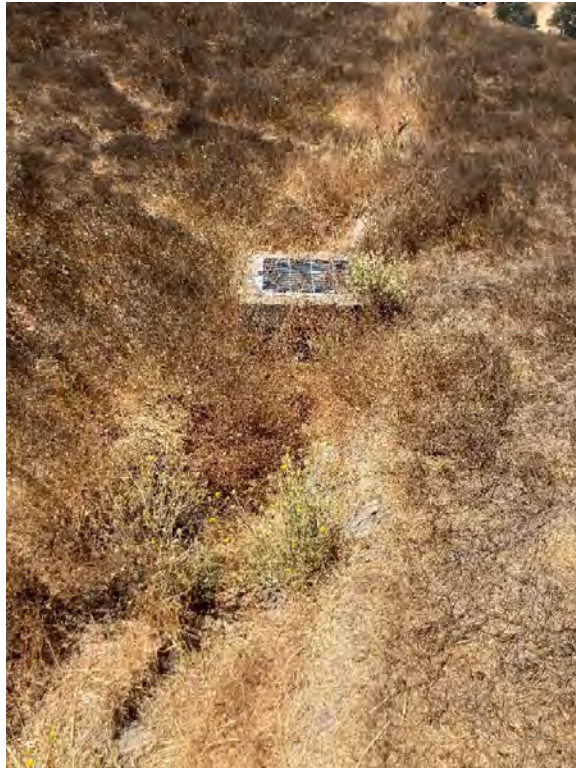
Photo 23. View of significant vegetative growth in and adjacent to the v-ditch.
