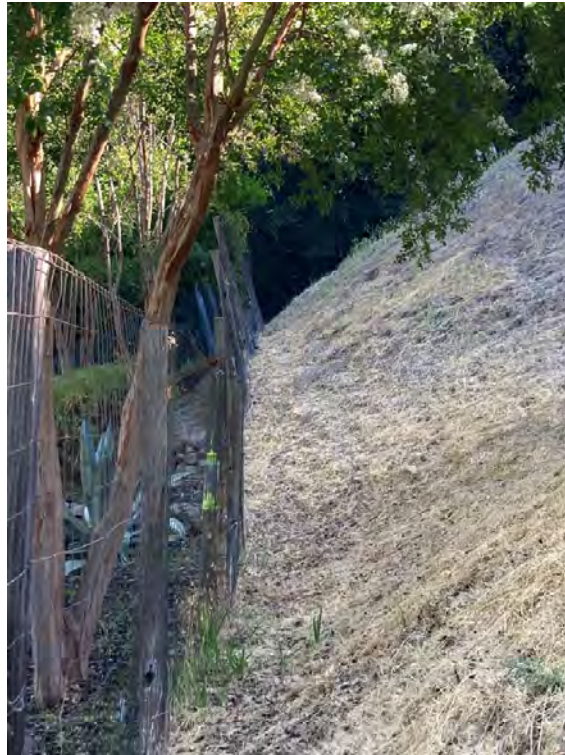
Photo 7. View of a shallow landslide impacting fence line to property below.
