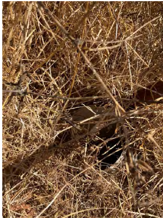
Photo 6. View of a subdrain cleanout riser missing a cap and debris allowed to enter the pipe.
