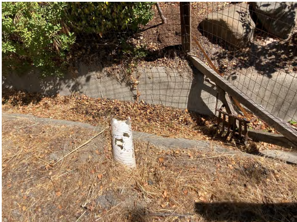
Photo 26. View of an outlet pipe into v-ditch, outlet pipe is damaged.
