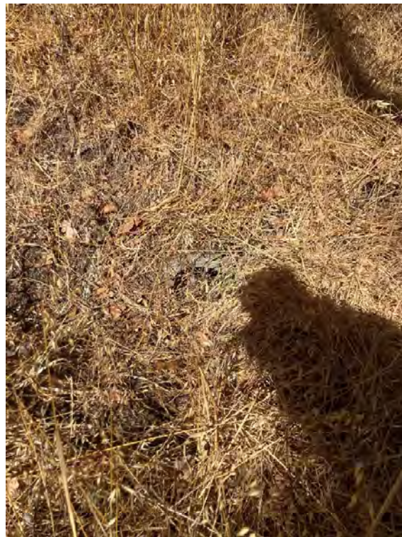
Photo 28. View of the partially blocked inlet for culvert pipe crossing under fire road south of 138 Windover Drive.
