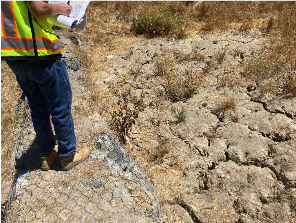
Photo 9. View of a basin behind gabion wall upslope of 124 Shadewell Drive full of sediment/debris.
