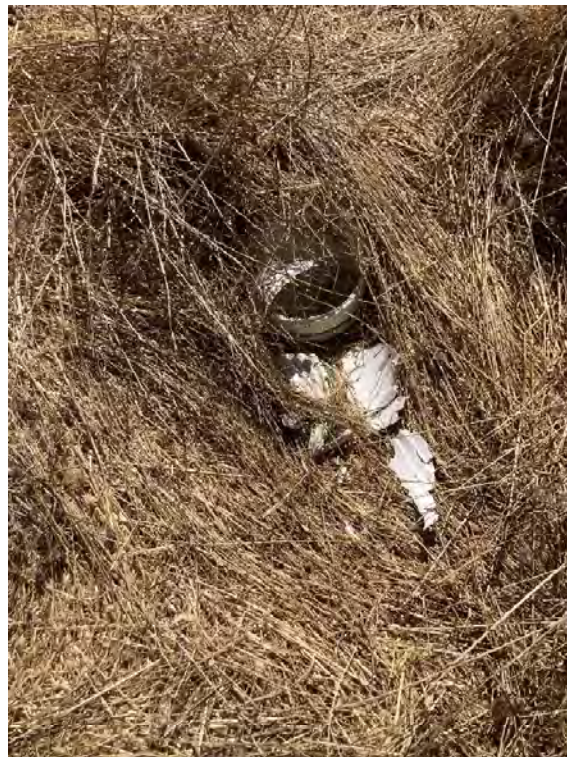
Photo 4. View of subdrain cleanout at ground level, hidden by vegetation, damaged, and missing a cap.
