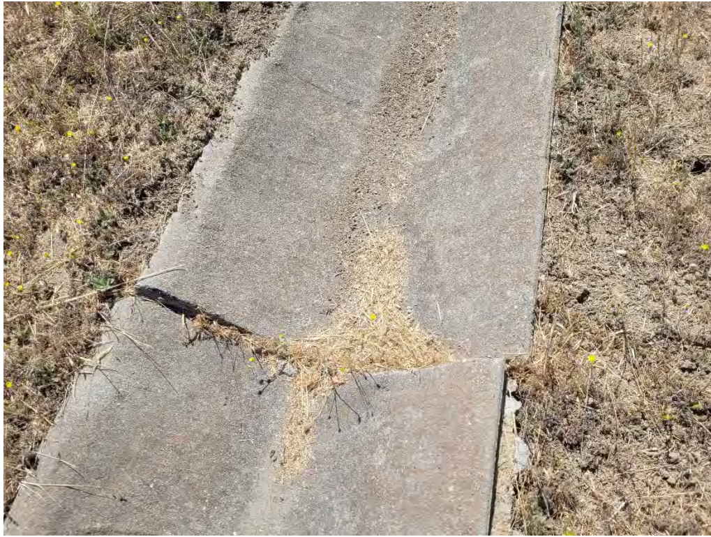
Photo 21. View of horizontal and vertical offsets with damming impacting flows of v-ditch.
