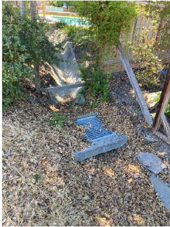
Photo 25. View of debris blocking drop inlet.
