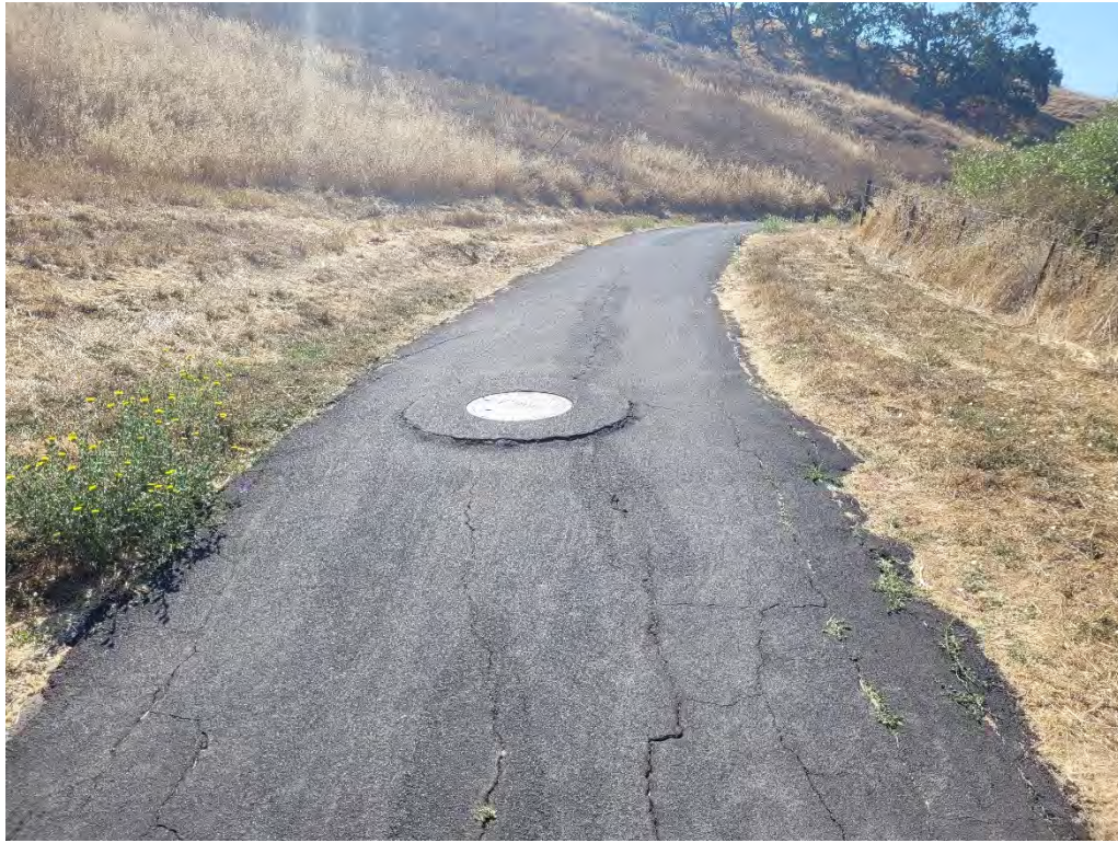
Photo 33. View of pavement cracking and settlement on Sunhaven Trail.
