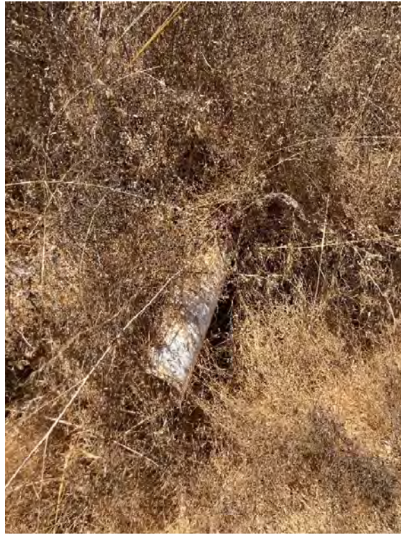
Photo 27. View of a subdrain outlet pipe blocked by vegetation.
