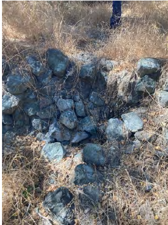
Photo 17. View of the failed stacked rock wall south of 138 Windover Drive.
