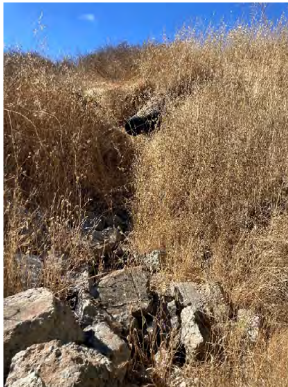
Photo 16. View of an 8-inch outlet pipe with downcutting along limits of rip rap.
