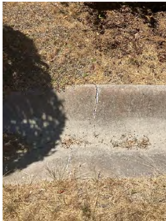
Photo 18. View of minor cracking of concrete-lined v-ditch.
