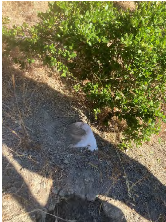
Photo 3. View of subdrain cleanout near ground level and obscured by vegetation.
