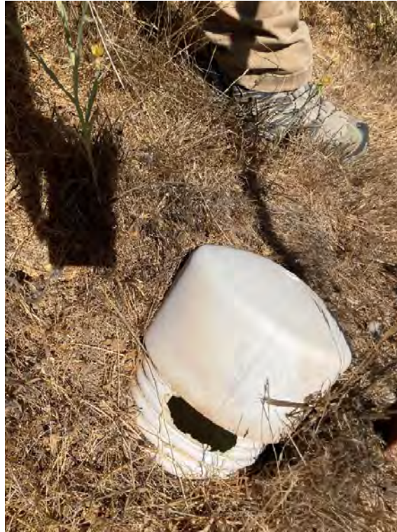
Photo 5. View of a damaged subdrain cleanout riser.
