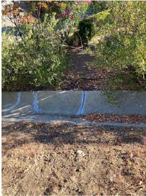
Photo 19. View of ongoing cracking at previous repair location within the v-ditch.
