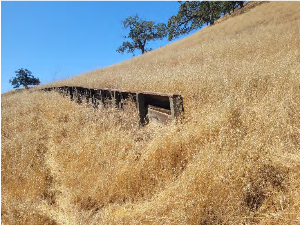
Photo 11. View of a failed wood catchment wall upslope of Saddleback Drive.
