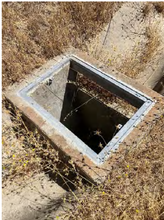
Photo 30. View of missing cover grate for drop inlet near 10 Hunters Terrace.
