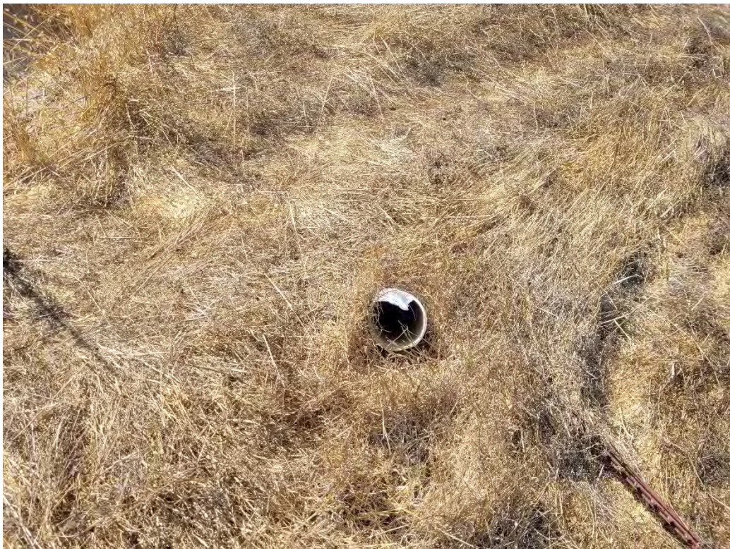
Photo 12. View of a damaged cleanout riser without a cap – debris observed within pipe and the T-post marker knocked over.
