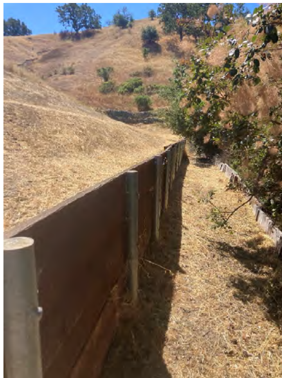
Photo 10. View of a leaning wall behind 124 Shadewell Drive.
