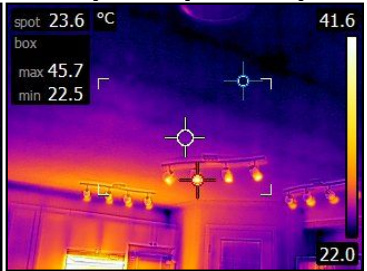
Kitchen Area Ceiling - Thermal Image
