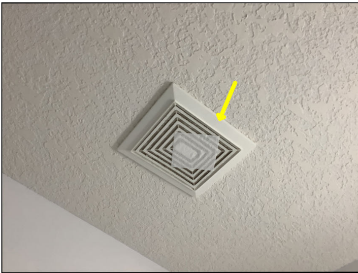
Main Level Bathroom- tested and working as required
