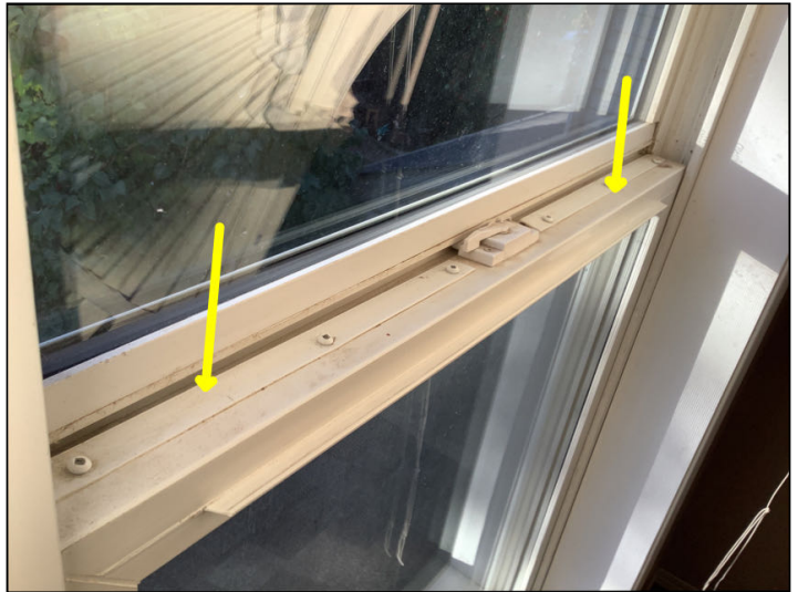
Clearly a draft issues at primary bedroom - seal and foam added - makes it hard to lock the window
