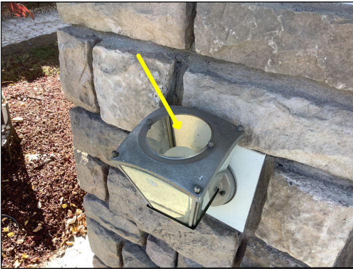
Garage lights - caps are missing - will allow rain into the units
