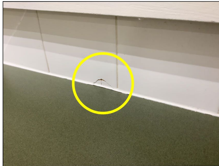
Damage tile - sink area
