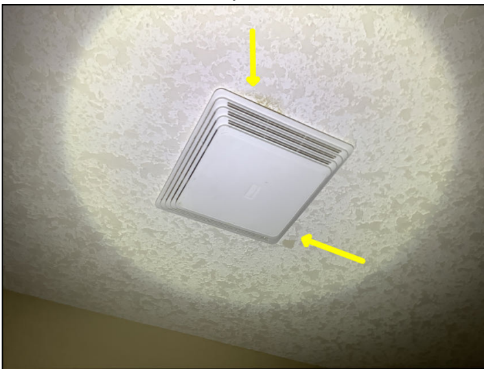
Family Bathroom- Staining noted to the fan surround.
