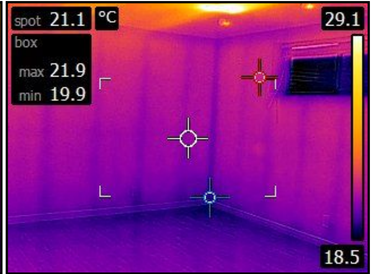
No major causes for concern below grade observed during the thermal scan.
