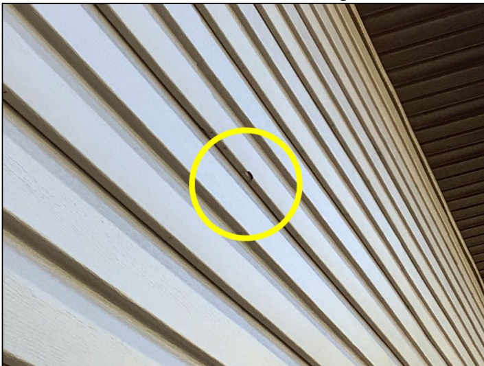
Areas of damage noted - right side
