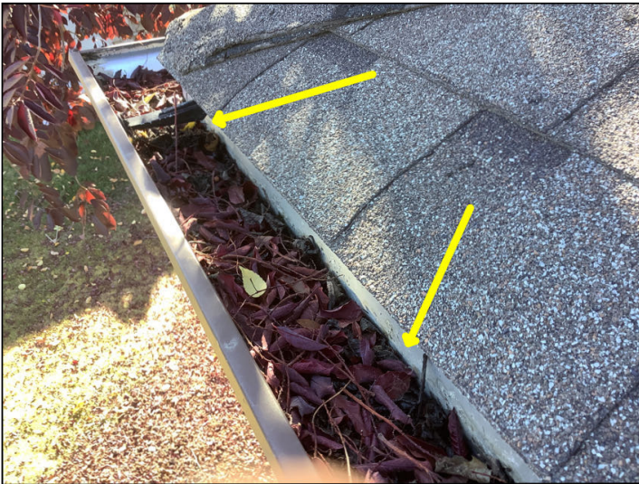
Clogged gutters noted. Suggest gutters be cleaned out as a part of a normal maintenance routine to ensure proper drainage.
