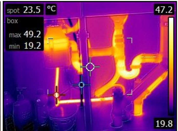
No leaks at traps or drains, water was run for some time to fully test for problems - a leak can develop at any time.
