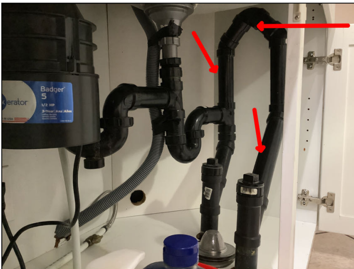
Very strange plumbing configuration under the sink - no venting - suggest plumber assess
