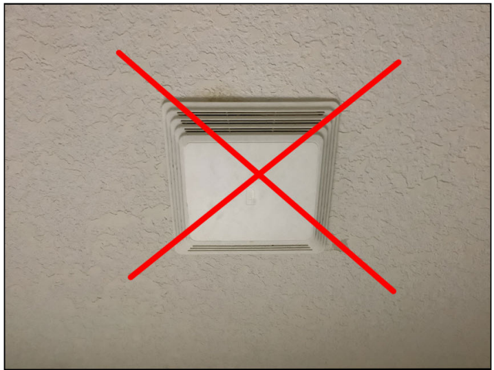
Poor draw noted on fan suggest repair/replace
