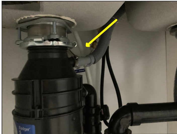
Dishwasher empties into the sinkerator
