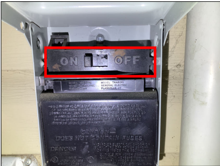
Power on - air conditioning failed to start
