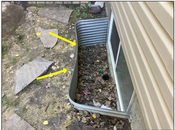
Window well under pressure
