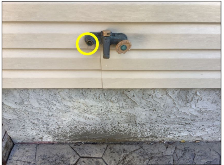
Rear faucet is missing one control
