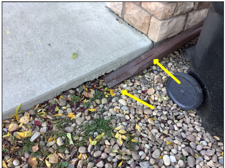
Re direct away from driveway
