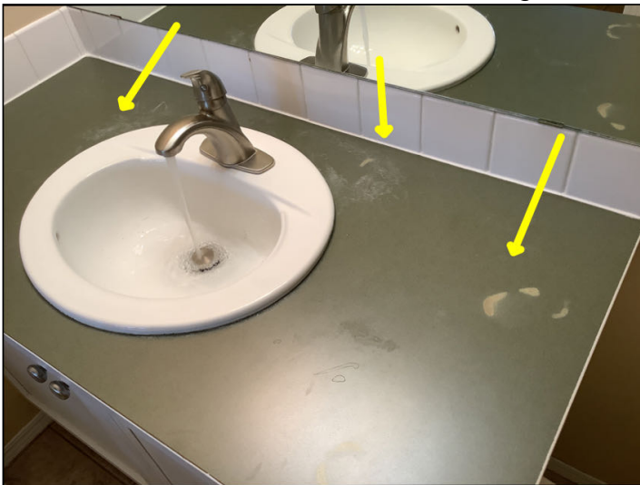
Cosmetic damage noted.
