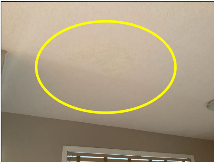
Stain noted - dry during thermal scan - suggest monitoring
