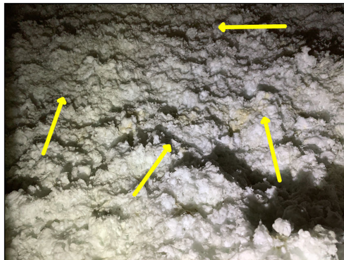
Staining in insulation would indicate past attic rain
