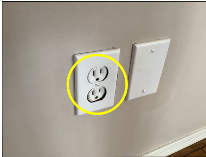
One receptacle requires attention in living room
