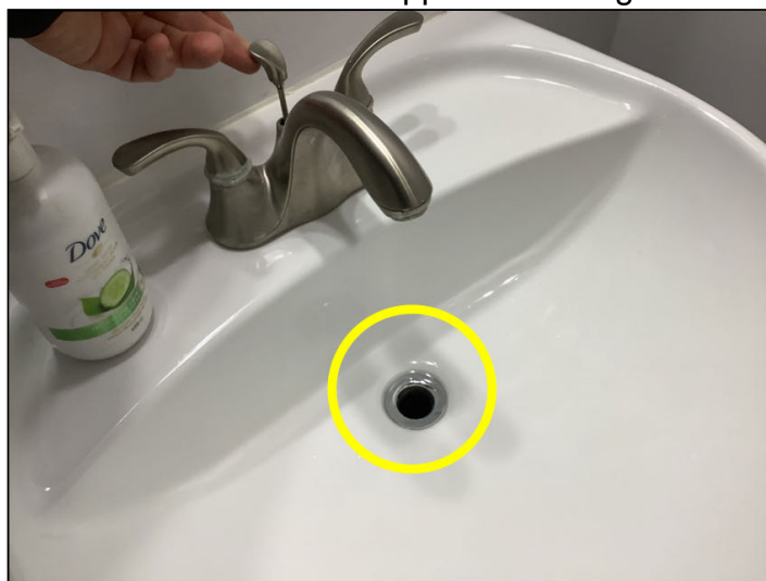
Main Level Bathroom - Stopper is missing at sink.
