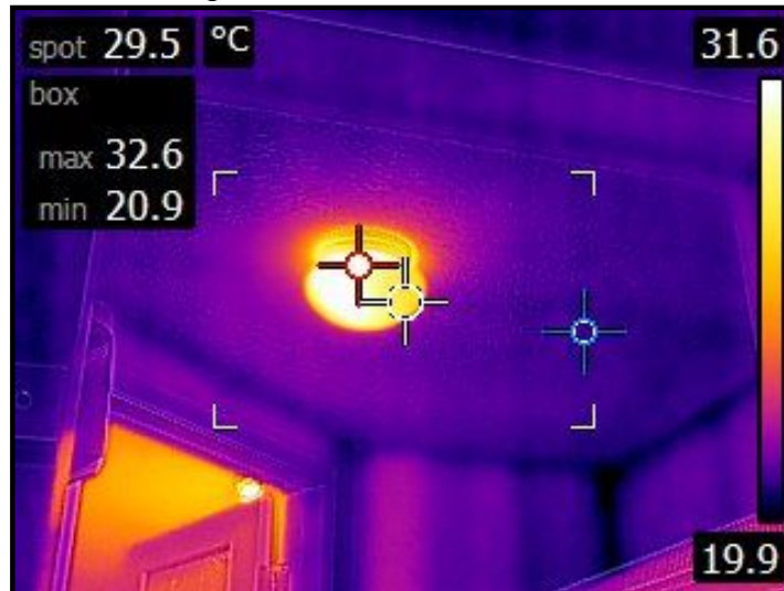
Pantry Area Ceiling - Thermal Image
