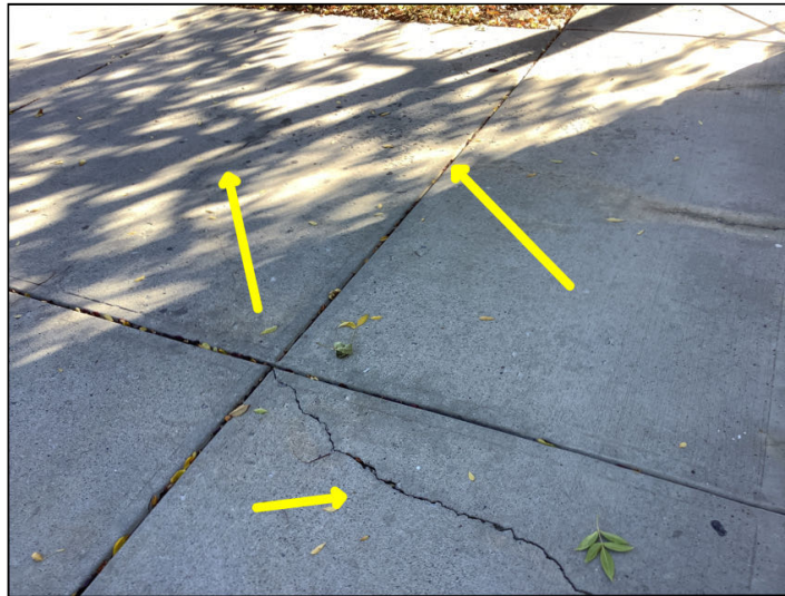
Common cracks and patching noted - over salting can damage concrete.
