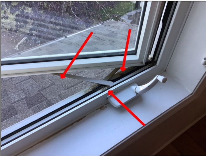
Bedroom 2 - window requires attention to open and close correctly - in an emergency situation egress would be hindered
