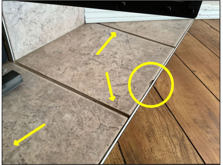
Re grouting required - damage tile noted
