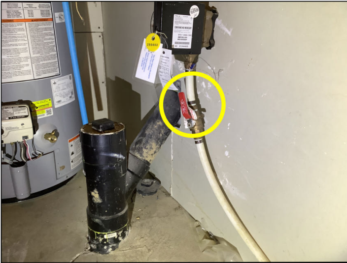
Main water shut off shown
