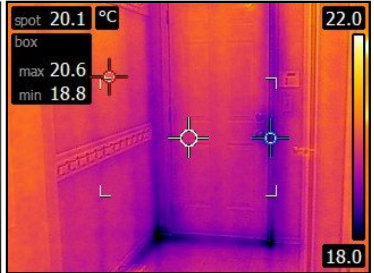
Mud Room - Thermal Image
