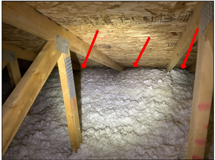
Someone has added batt insulation around the perimeter blocking the soffit vents
