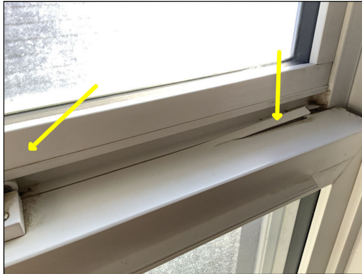
Trim damaged at window in en suite
