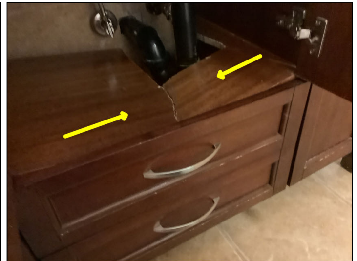
Repairs required to cabinets
