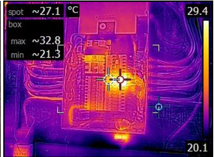
Thermal Image of panel - No issues during inspection
