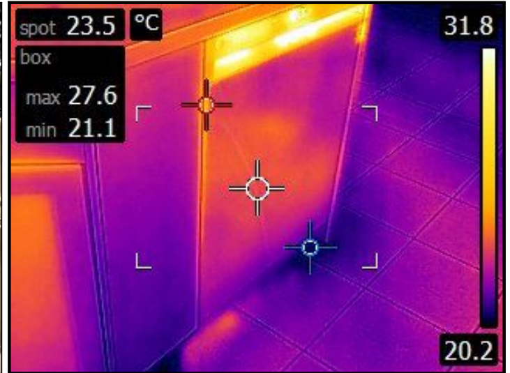
Thermal image showing no leaks after full cycle
