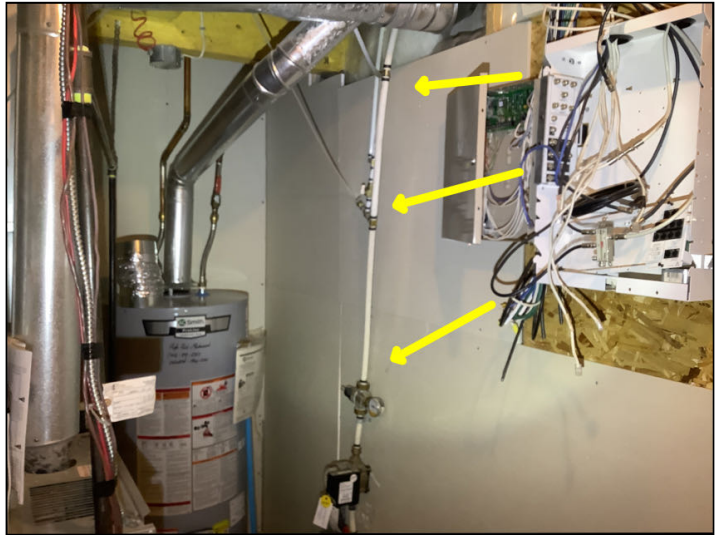
Service lines are loose - recommend securing as required.
