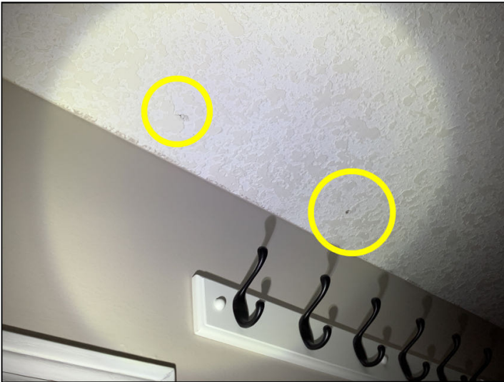
Drywall pops occur usually from the studs drying and twisting. The cure is simple, re screw above and below the "pop" within 1 inch, turn the old screw in by hand, then mud.
