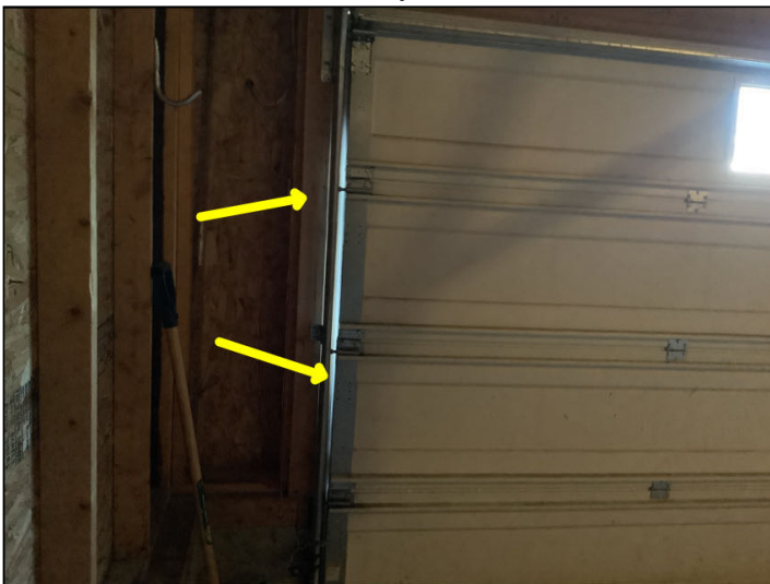
Weatherstripping does not create a good seal either side of the door
