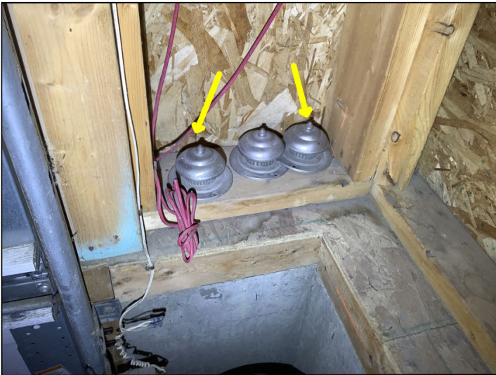
Light caps in garage area
