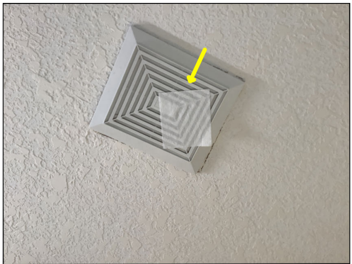
En Suite To Primary Bedroom- tested and working as required
