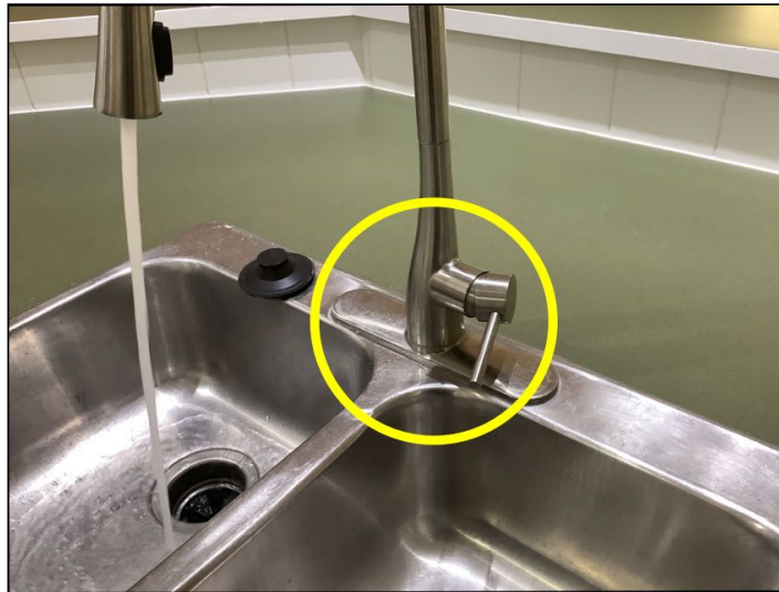
Faucet is loose - Recommend securing.
