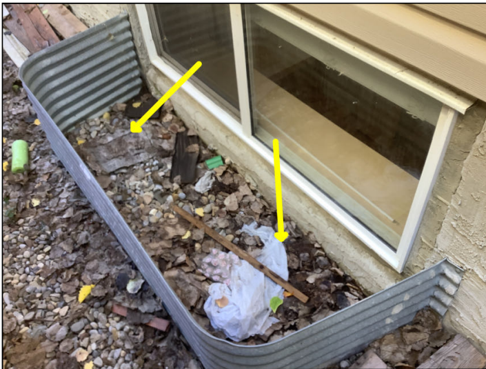
Keep window wells clean and clear
