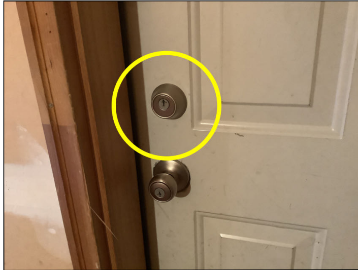
Top lock installed upside down
