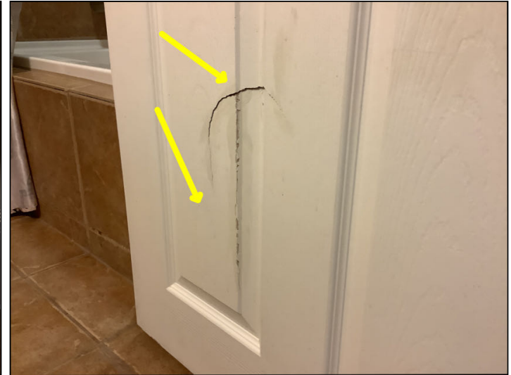
Basement bathroom - damaged door
