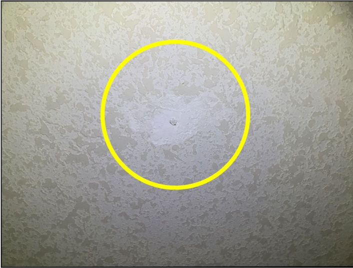
Cosmetic damage noted at bedroom ceilings
