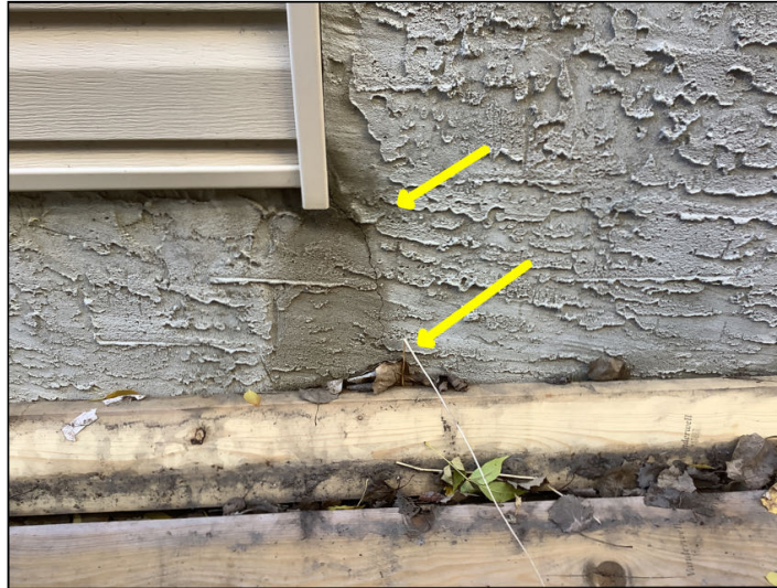
Cracks noted - right side
