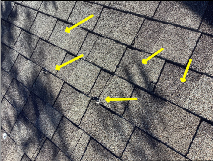
Damage at garage appears to be from roofers ladders
