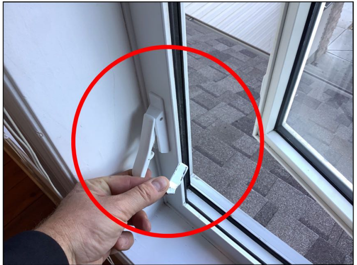
Bedroom 3 - Window locks are not operation/broken, this poses a security issue.
