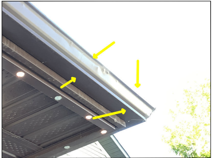
Hail damage noted to gutters - cosmetic only and does not effect the performance.
