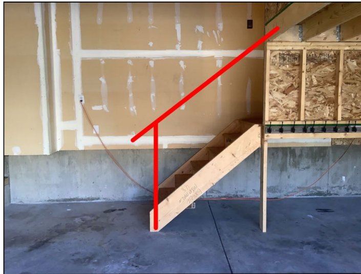
Handrail is required where 3 or more stairs are in place
