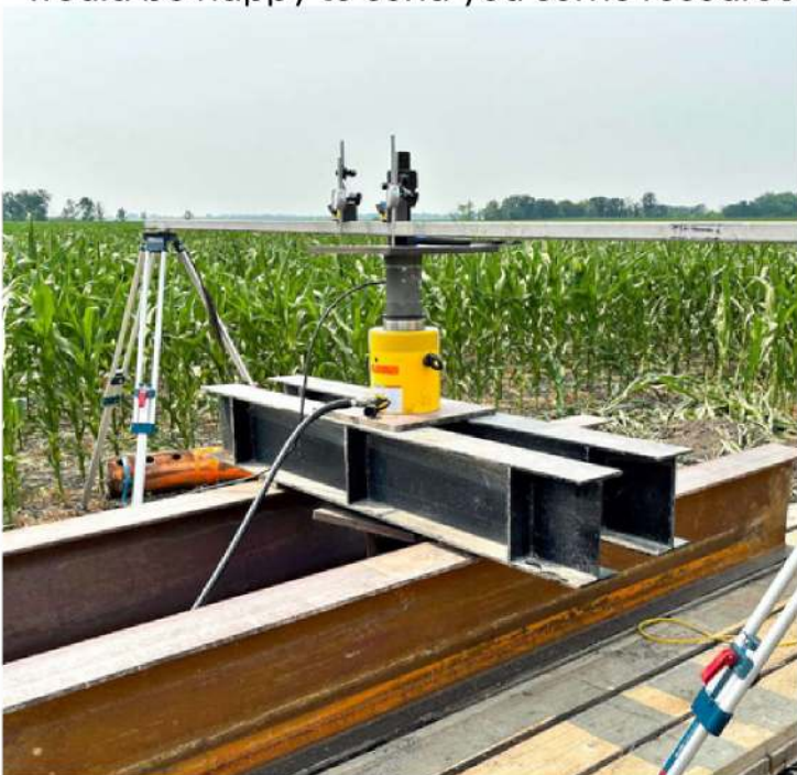
A hydraulic jack attached to a steel test-rig applies force to test the compressive resistance of a helical pile.
