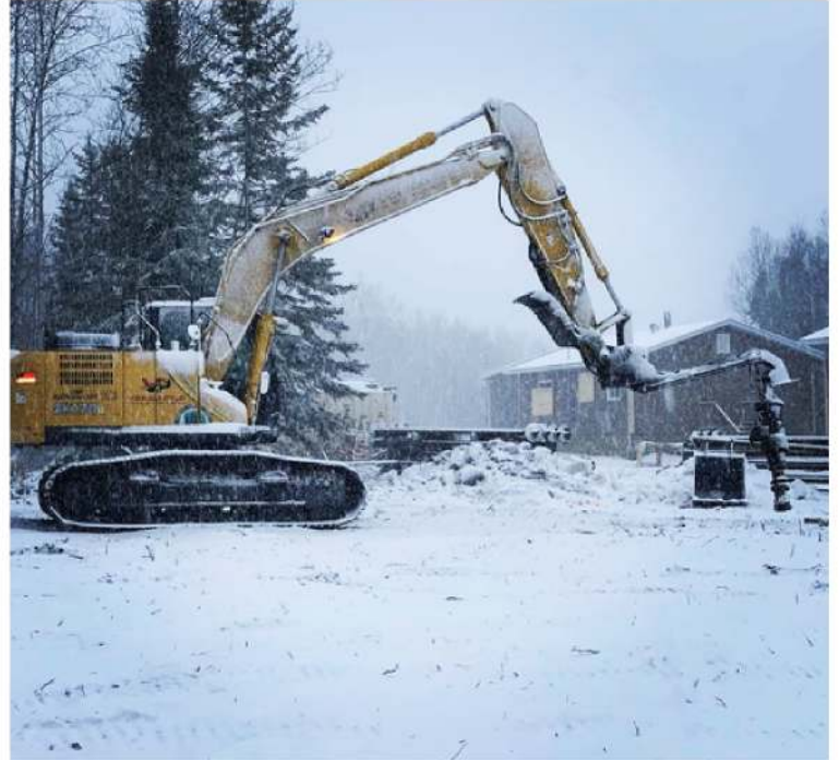
Helical piles can be installed in a range of weather conditions, including a snowstorm.
