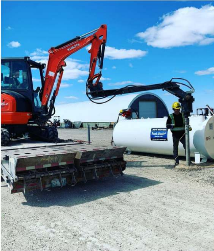
This Kubota mini-excavator was able to install these piles for protective bollards right from the trailer.
