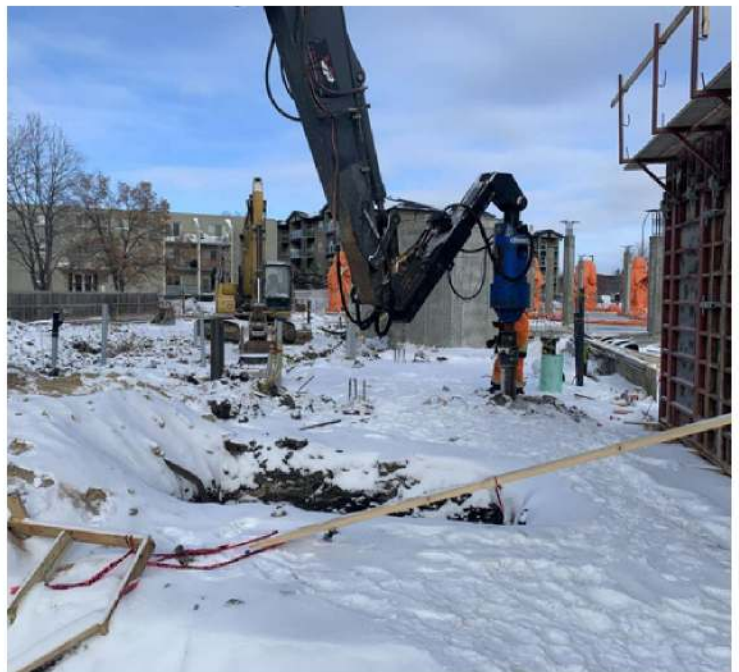
Pre-existing concrete walls made driven piles infeasible. Helical piles install with zero disturbance, which made them a strong choice on this sensitive jobsite.
