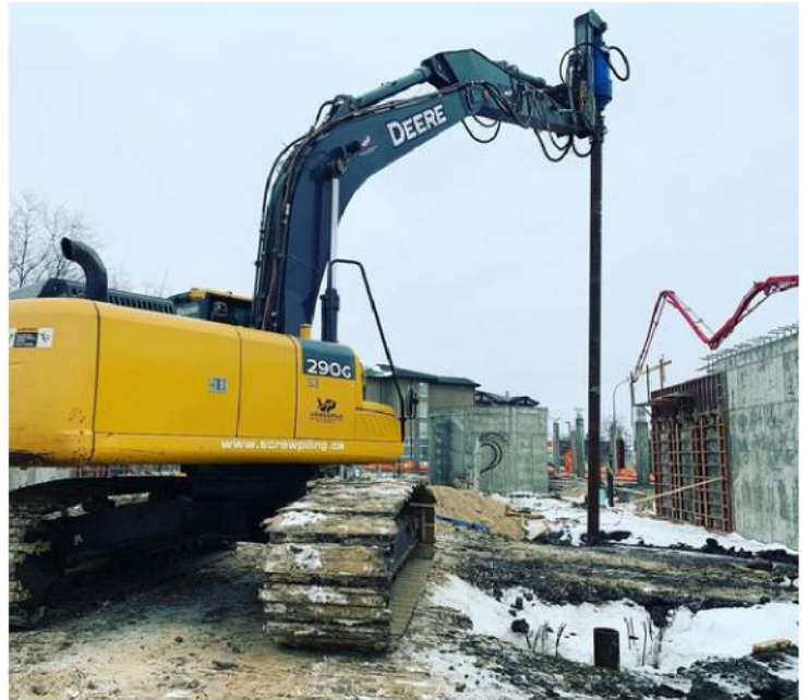
A Deere 290G excavator installing high-capacity helical piles for a 5-storey multi-use project.
