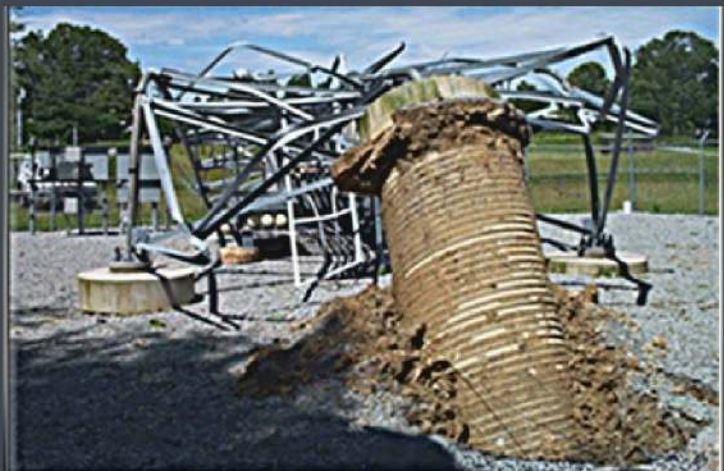
This transmission tower foundation failed due to uplift forces from frost (Image courtesy of "Adfreeze Forces on Lightly Loaded Pile Foundations of Solar PV Farms in Cold Regions")
